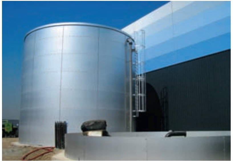
At the Chaponnay warehouse, offices are supplied with electricity from photovoltaic panels installed on sprinkler tanks
